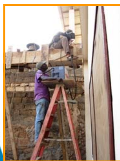
Using the small welder Jason got on Craig's List to secure of the supports for the solar system onto the front of Guest House
