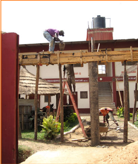
The cement is mixed in our amazing cement mixer and then dumped into a wheelbarrow. After that they scoop it into buckets and hand them up to be poured into the wooden forms
