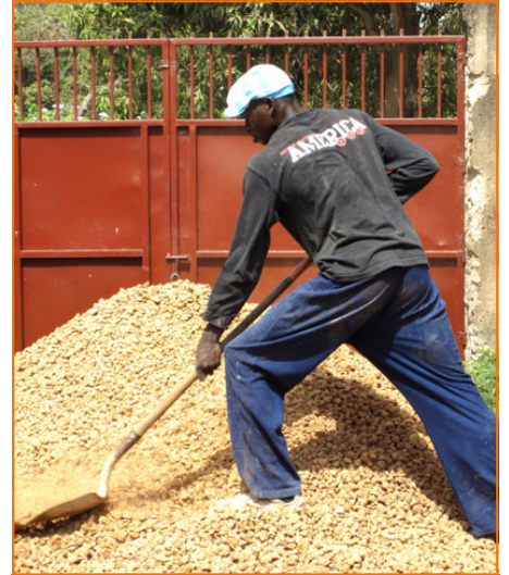
Filling the cement mixer with just the right amounts of gravel, sand, water, and cement powder
