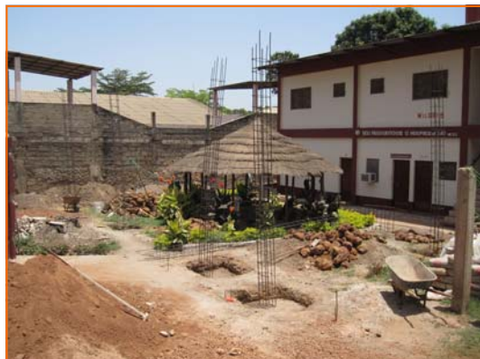
After digging and pouring the cement footings this is what the structure looked like when we started
