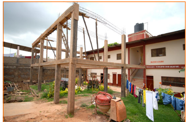
As you can see we are making tons of progress, and as soon as we pour the remaining columns to connect it all together Jason can start building the grid on top that will hold the panels
