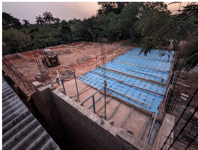
The new shop is divided into a pair of 20'x60' wings on either side of a central 40'x60' fabrication area. We're working to quickly complete one of the wings, seen here ready for the remaining five sections of slab to complete its floor.
