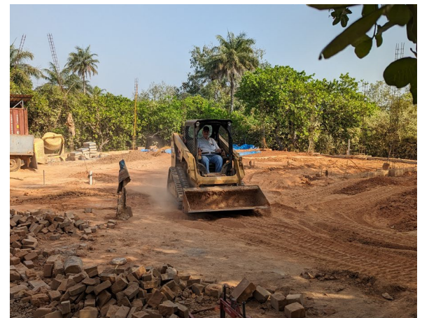
Jim R. spent most of the week digging dirt out of the mine and filling the shop footprint, a task I had been working on and thought would never end!
