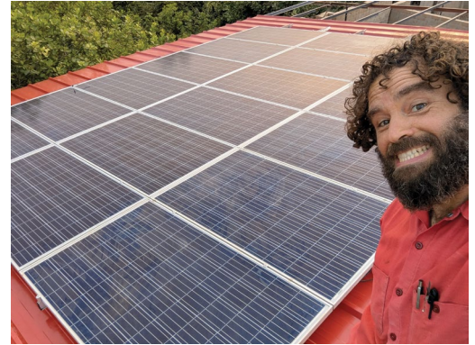
Though we've had solar panels in temporary mounts since almost the beginning of construction, this month we got to mount the first panels in their permanent location. This section is about a third of the eventual system that will run the shop and site.
