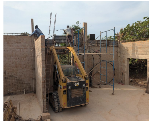
Blocks, columns, and bond beams continue to go up. The shop is advancing!
