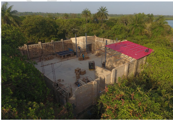
The new shop construction is marching along, with its first roof section and walls getting taller!
