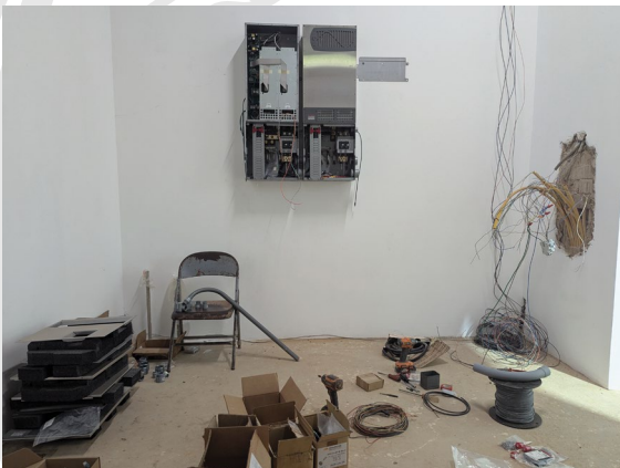
Five years in the making: the solar system electronics begin permanent installation!
