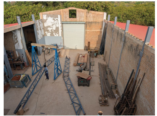
The central section of the new shop is playing both doctor and patient as we build the roof trusses to cover it, inside it.
